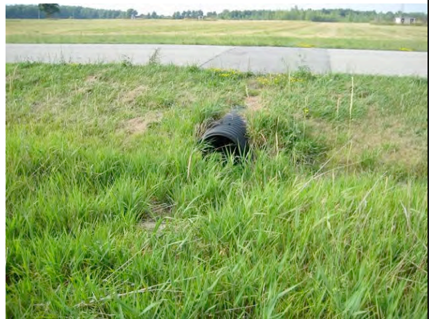
Image 4: View of plastic/rubber culvert under Sobie Road, for north-south unnamed drainage located immediately west of Subject Lands.
